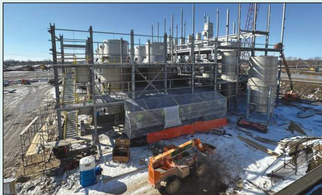
STRUCTURAL STEEL rises last month at the Michigan Sugar Company's $75 million de-sugarization plant in Bay City. Iron Workers Local 25 members on the job are employed by Dobson Industrial and Monarch Welding.
