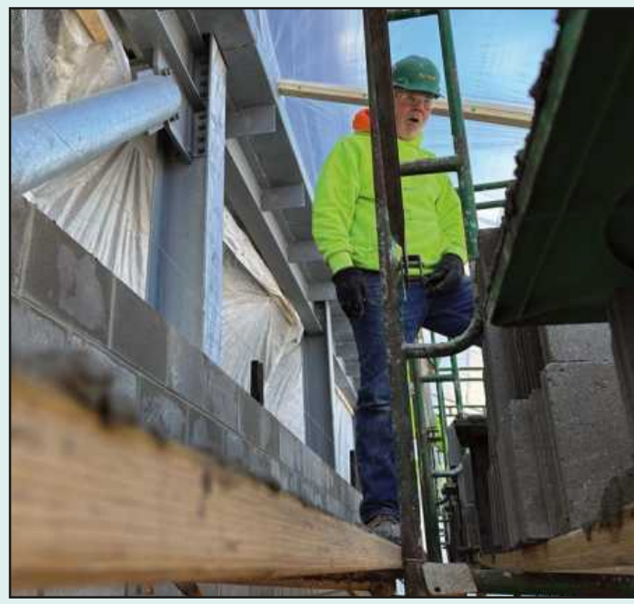
SETTING BLOCK at the Michigan Sugar Co. plant in Bay City is Ed Morse of Bricklayers and Allied Craftworkers Local 2. He's employed by Pumford.
